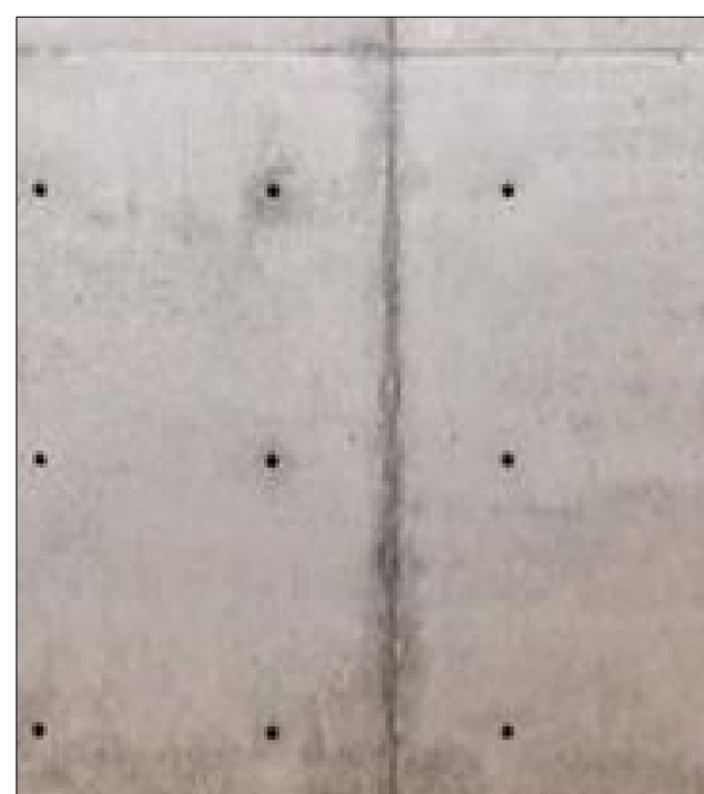
C - OFF-FORM CONCRETE
